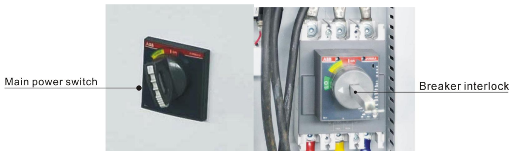
Picture 4-2: Main Power Switch
