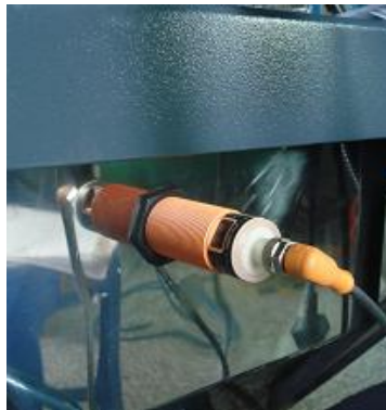
Picture 4-32: Level Switch on storage Tank
