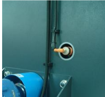
Picture 4-31: Level Switch on Mixing Tank
