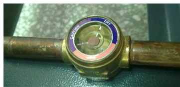
Picture 2-33: Refrigerant Indicator
