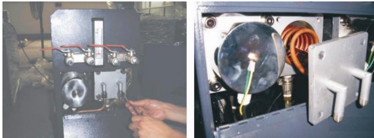
Picture 6-10: Cooling Pipes 2
