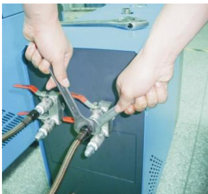
Picture 3-2: Mould and Water Coupling 1
