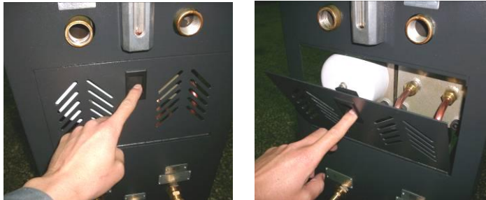
Picture 6-6: Pipe Heater 1
