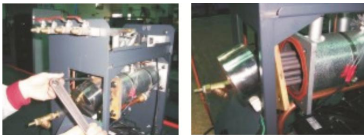
Picture 6-8: Pipe Heater 3
