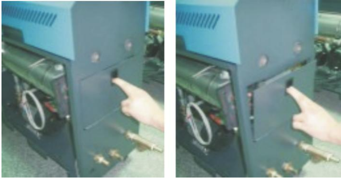
Picture 6-6: Pipe Heater 1
